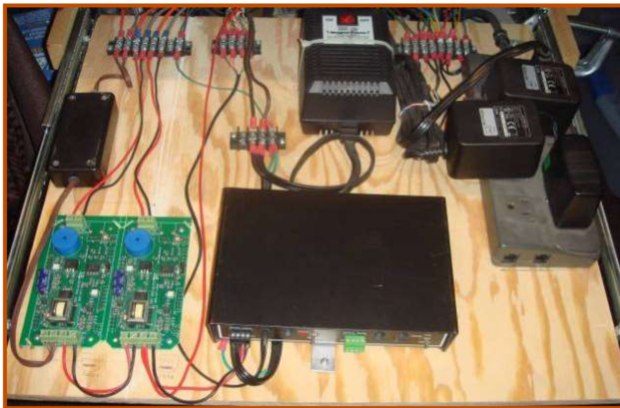
Glendale/Mesa Booster Board. There are six booster boards measuring 20in x18in.
